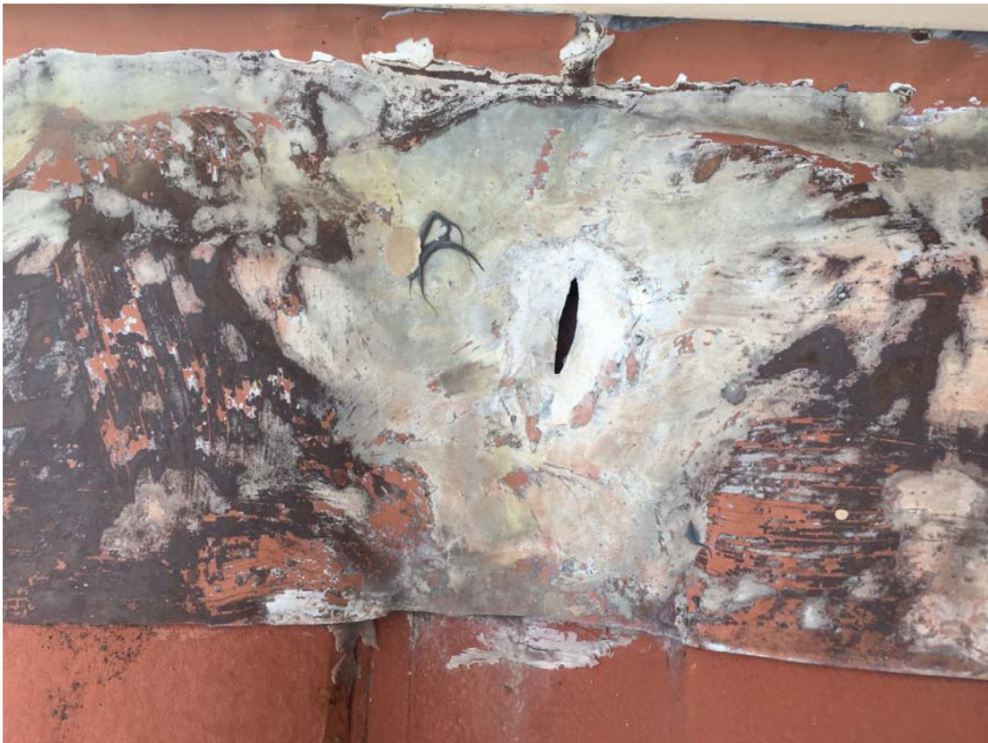
PHOTOGRAPH 9. LEAD FLASHINGS AT THE HEADWALL HAVE A FEW TEARS OR PUNCTURES.
