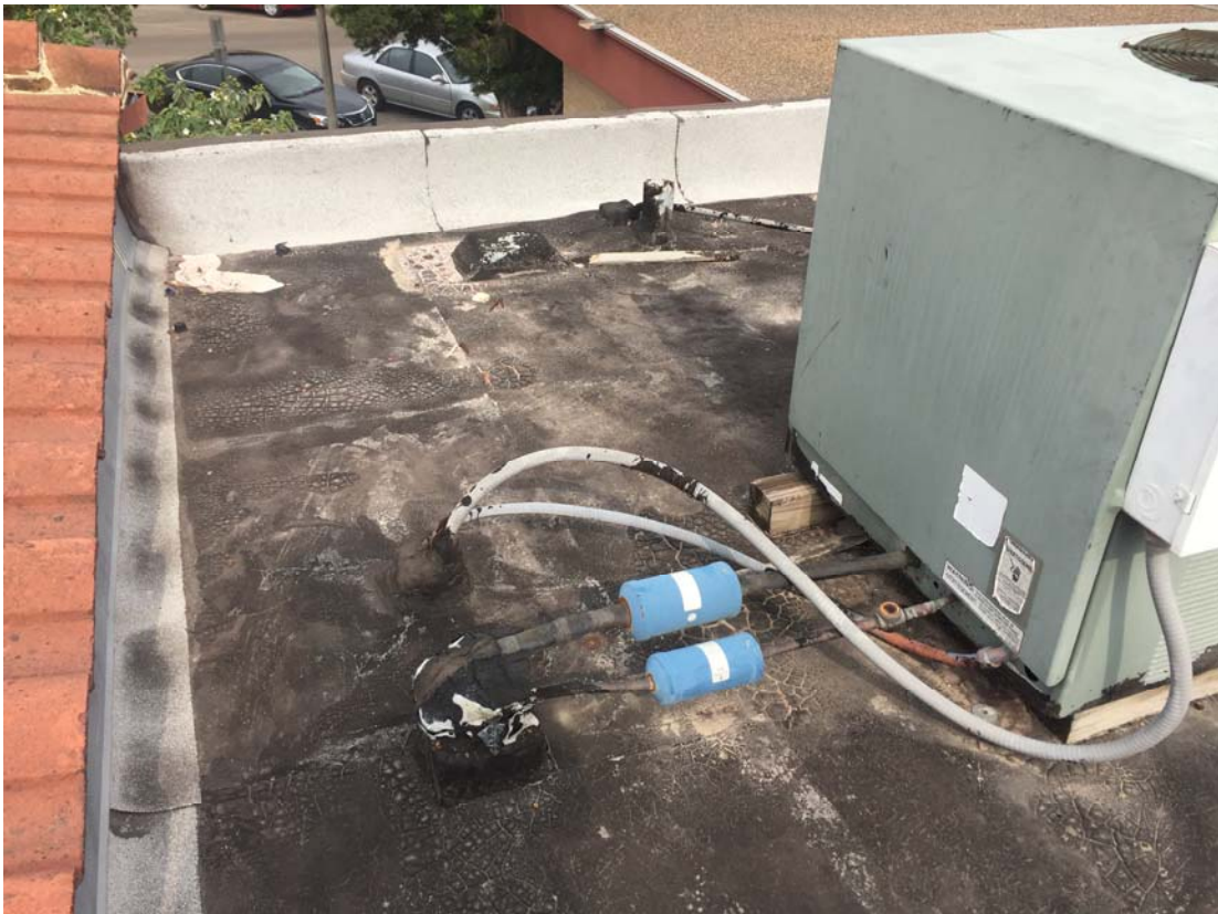
PHOTOGRAPH 18. BUR ROOF AT THE NORTH SIDE OF AREA 3 TILE ROOF IS IN FAILURE MODE AS WELL DUE TO THE SAME CONDITIONS NOTED ABOVE REGARDING THE SOUTH SIDE.
