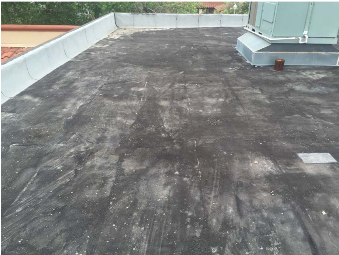
PHOTOGRAPH 10. BUILT-UP ROOF LOW SLOPE ROOF AT THE THEATER/A.V. (AREA 3). SYSTEM IS SEVERELY DETERIORATED AND IN FAILURE MODE. AGAIN, THERE ARE NO COPING CAP PROTECTING THE TOP OF THE PARAPETS. CORE CUTS REVEALED THE METAL DECK IS RUSTED AND CORRODED FROM WATER PASSING THRU THE SYSTEM WHICH IS NO LONGER CONSIDERED WATERTIGHT.
