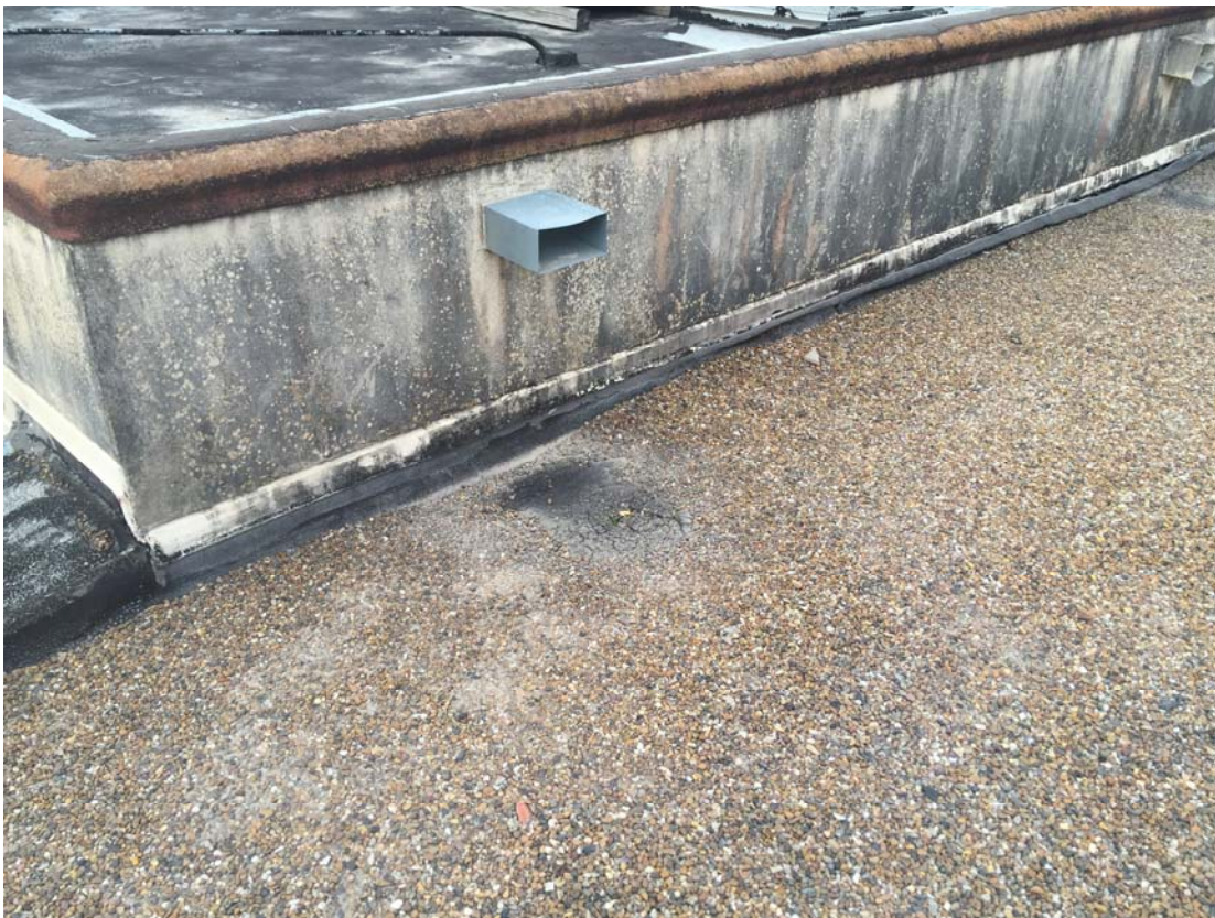
PHOTOGRAPH 17. EXPANSION JOINT TRANSITION TO THE STUCCO RISE WALL ADJOINING AREA 3 AND 4 IS FAILING. NO COPING CAP IS ATOP THE PARAPETS. AREA 4 BUR ROOF WITH GRAVEL SURFACING HAS SURPASSED ITS SERVICEABLE LIFE AND IN FAILURE MODE.
