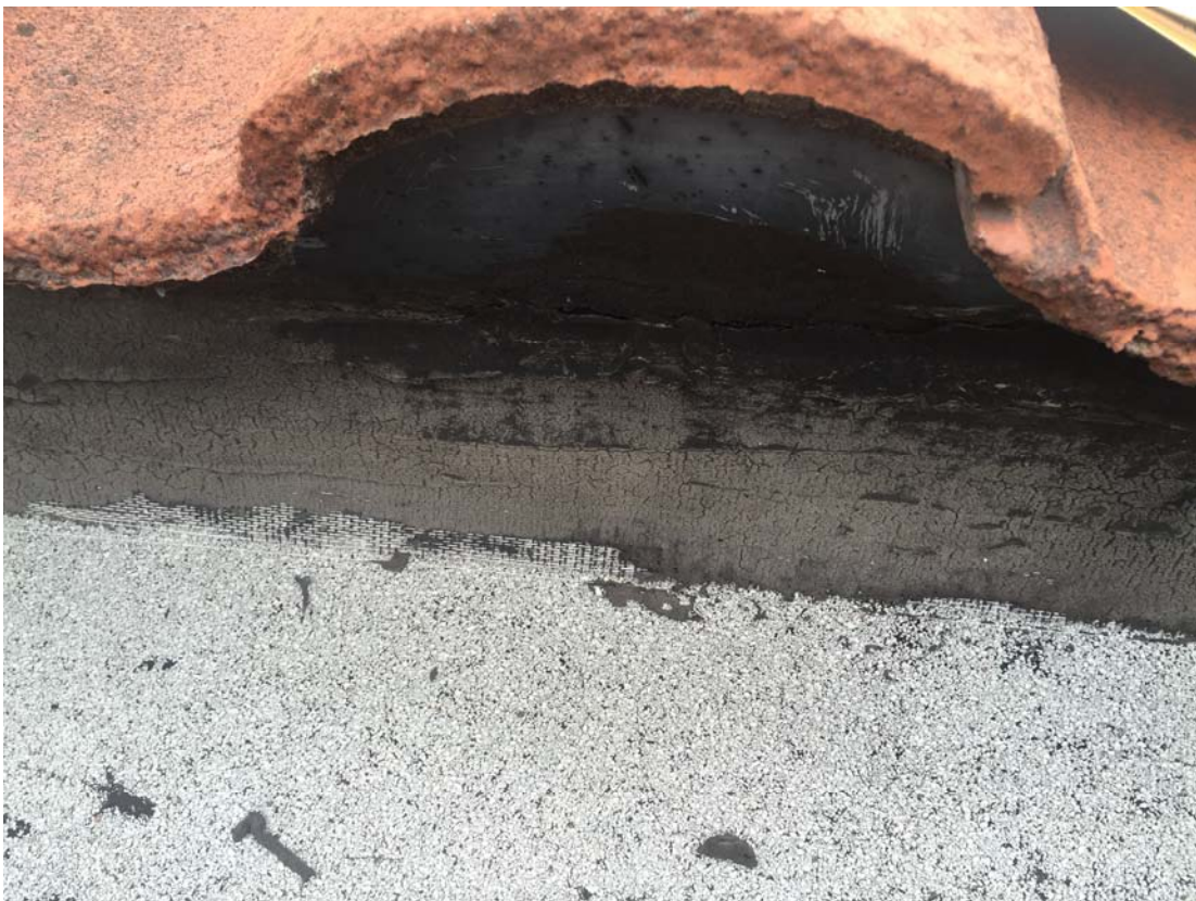
PHOTOGRAPH 16. THE TILE EAVES TRANSITION TO THE LOW SLOPE ROOF BELOW ARE IMPROPERLY INSTALLED. TOP OF THE BASE FLASHING MEMBRANE IS OPEN OR IMPROPERLY SECURED AND SEALED THROUGHOUT CREATING A SEVERE LEAK SOURCE.
