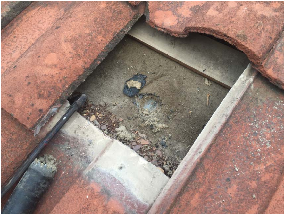
PHOTOGRAPH 13. THE TILE ROOF AT THE THEATER CONSISTS OF A METAL DECK, PERLITE INSULATION, MOPPED PLY FELTS AND THE CONCRETE TILE ROOFING SYSTEM. WHEN THE WOOD BATTENS WERE SECURED TO THE METAL DECK BELOW, THEY ACTUALLY CREATED A LEAK SOURCE DUE TO THE ASPHALT ADHESIVE BEING HARDENED ONCE IT DRIED. THE ASPHALT MOPPING IS NOT SELF SEALING AROUND THE FASTENER SHANKS.
