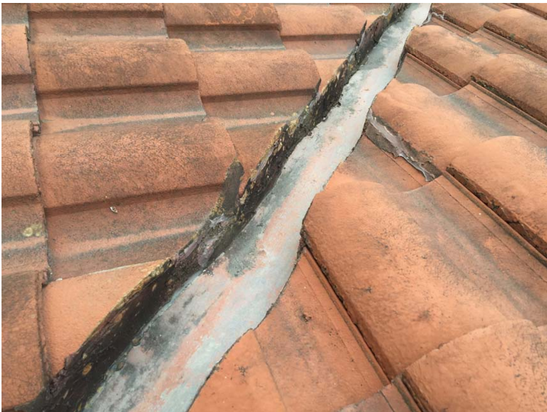
PHOTOGRAPH 6. VALLEYS APPEAR TO BE NARROW WITHOUT A DIVERTER. THE BLACKENED MORTAR INDICATES MOISTURE WICKED INTO THE MORTAR AND MOST LIKELY BEHIND IT AS WELL.
