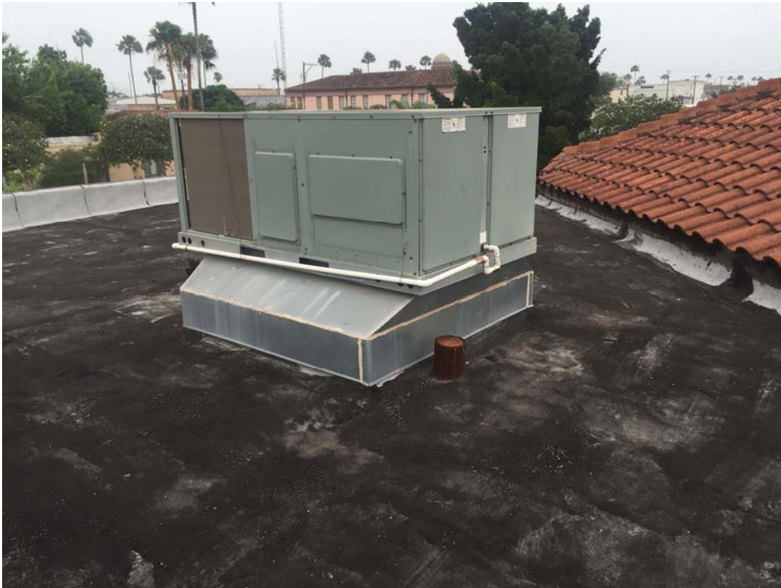
PHOTOGRAPH 11. HVAC EQUIPMENT CURBS APPEAR TO BE RETRO-FITTED AND IMPROPERLY FLASHED TO THE ROOFING SYSTEM.
