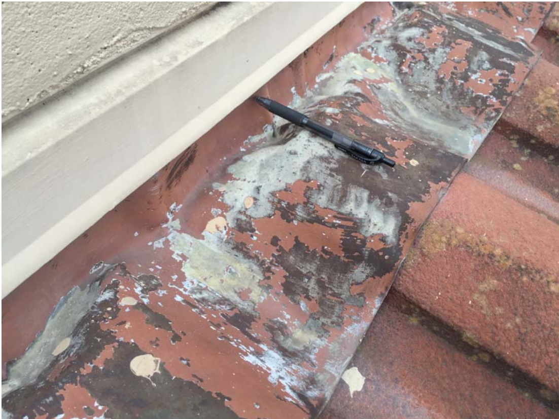
PHOTOGRAPH 8. LEAD FLASHINGS AT THE TILE HEADWALL ARE DEFORMED, CREATING A DEPRESSION BEHIND THE HEAD OF THE TILE. WHEN THERE IS A LAP NEARBY, MOISTURE WILL ENTER THRU THE LAP AND SUBSEQUENTLY BENEATH THE TILE.
