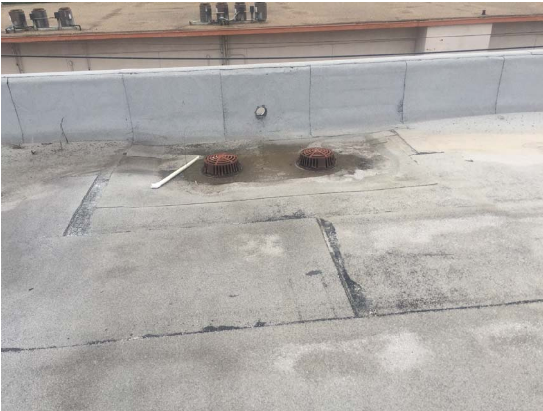
PHOTOGRAPH 3. AREA 1 APPEARS TO BE UNDER DRAINED WITH INSUFFICIENT EMERGENCY OVERFLOW DRAINAGE. ALSO THERE IS NO COPING CAP PROTECTING THE TOP OF THE PARAPET WALL.
