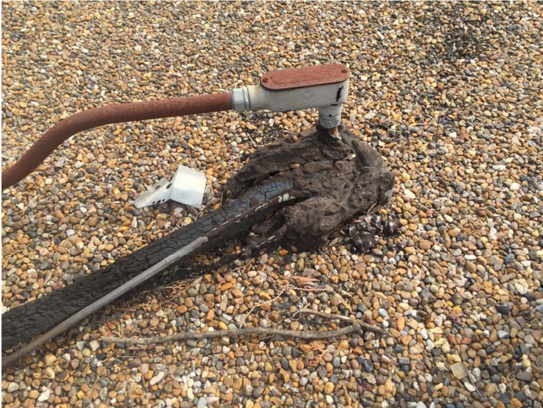
PHOTOGRAPH 21. ROOF PENETRATIONS ARE IMPROPERLY APPLIED AND SEALED AND HAVE NOT BEEN MAINTAINED.
