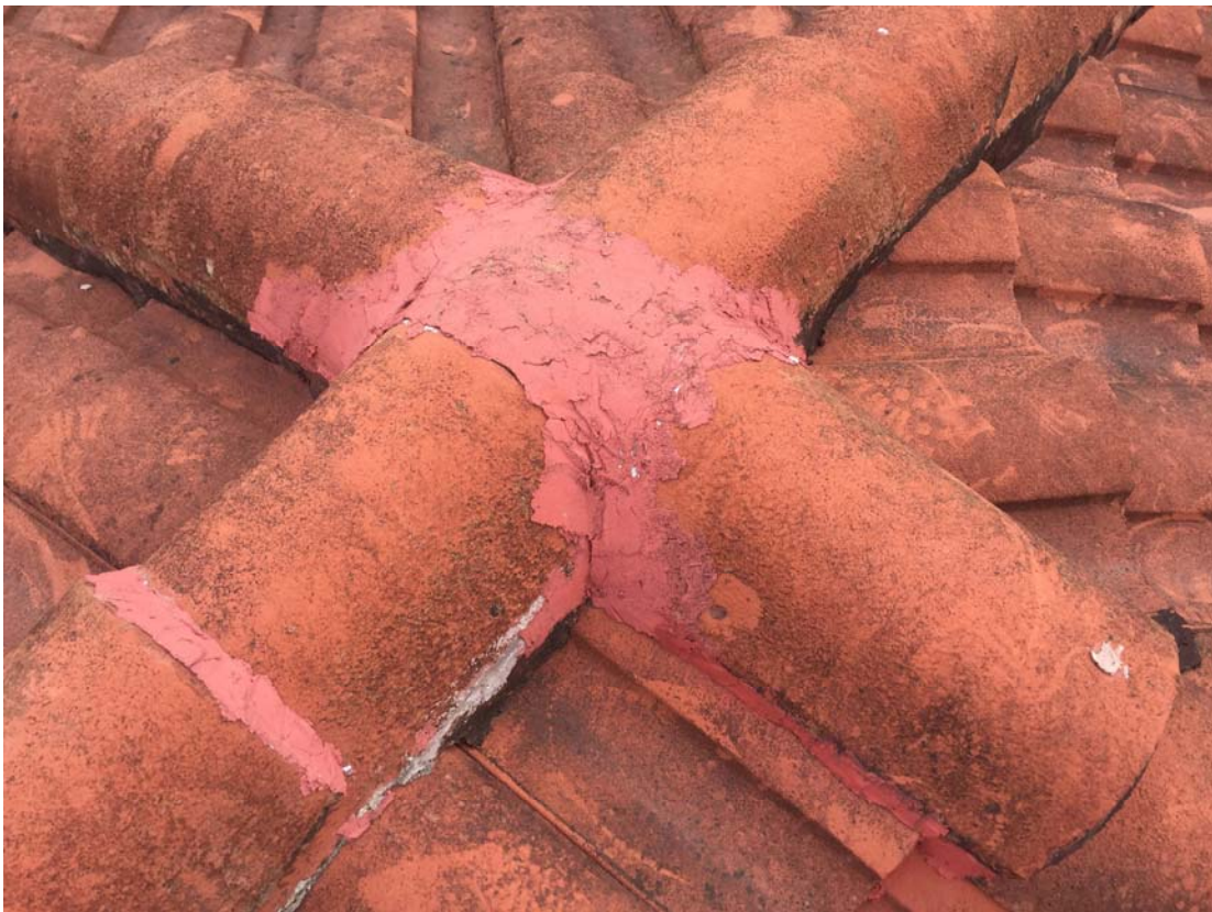
PHOTOGRAPH 14. THE TILE HIPS, RIDGE, AND APEX TRANSITIONS HAVE DETERIORATED MORTAR. IT APPEARS THEY HAVE BEEN REPAIRED SEVERAL TIMES OVER THE YEARS BUT WITHOUT LONG TERM SUCCESS.
