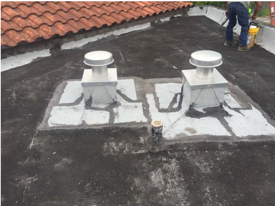
PHOTOGRAPH 12. THESE EXHAUST FANS APPEAR TO HAVE BEEN RECENTLY INSTALLED WITH PROPER CURBS AND BASE FLASHINGS.
