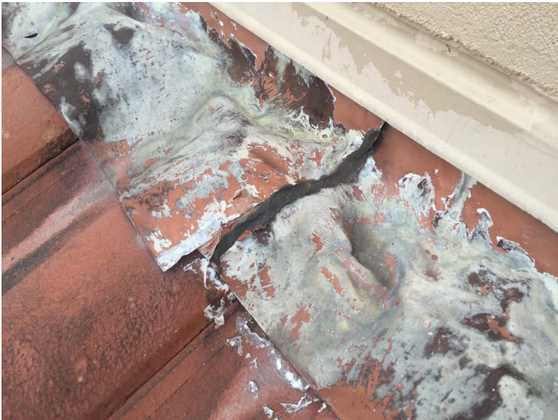
PHOTOGRAPH 7. LEAD FLASHING LAPS AT THE TILE HEADWALL ARE LACKING A PROPER SEAL OR ARE OPEN.
