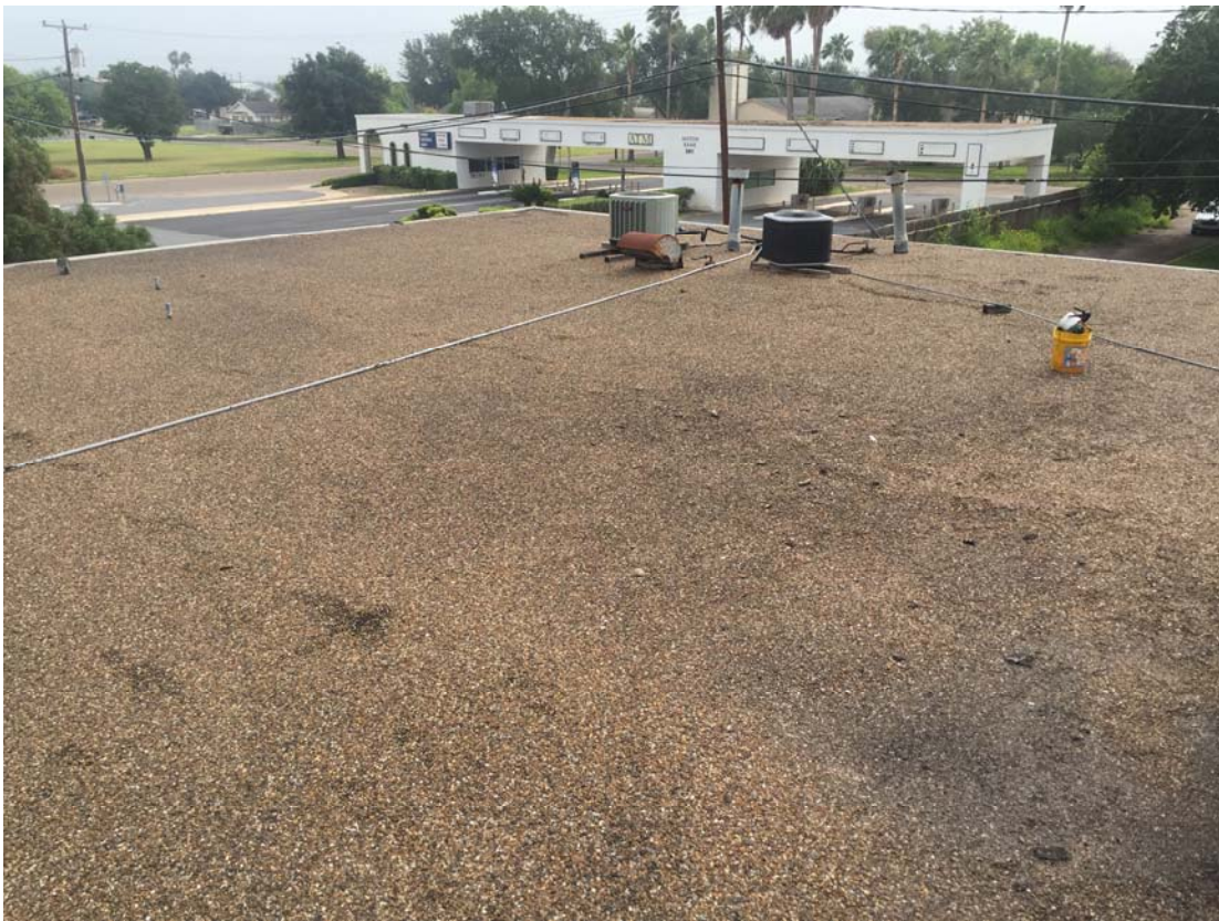
PHOTOGRAPH 19. AREA 4 BUR ROOFING SYSTEM WITH GRAVEL SURFACING HAS SEVERELY OXIDIZED AND IS CONSIDERED TO BE IN FAILURE MODE.
