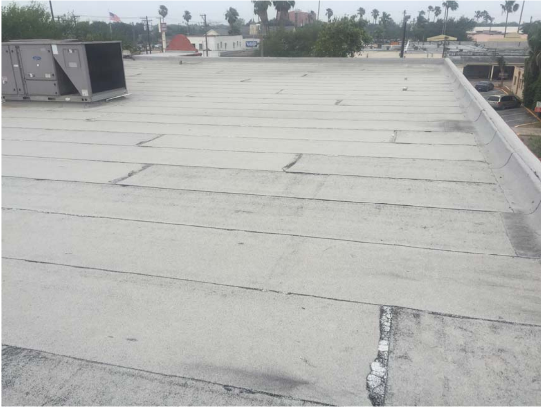
PHOTOGRAPH 1. VIEW OF SBS MODIFIED BITUMEN ROOFING SYSTEM OVER AREA 1 WHICH IS THE NEW LIBRARY MAIN BUILDING. MEMBRANE IS STARTING TO SHOW SOME OXIDATION AND GRANULAR EROSION.
