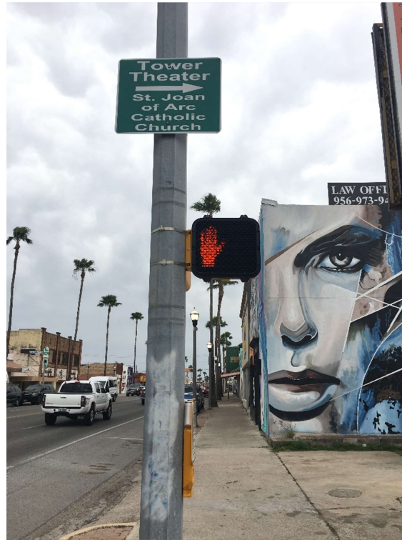
Figure 25: Upgraded LED Pedestrian Indicator
