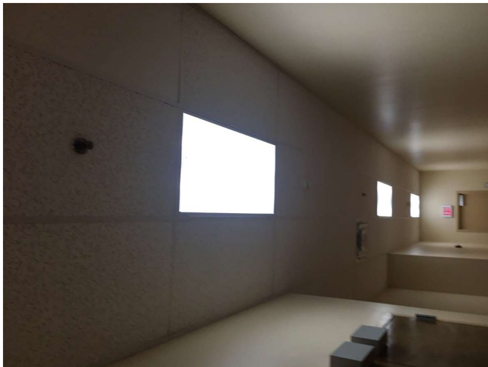
Figure 24: 2 x 4 LED Fixture in hallway at City Hall
