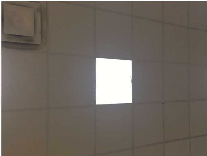
Figure 15: 2x2 LED Light Fixture at Public Library
