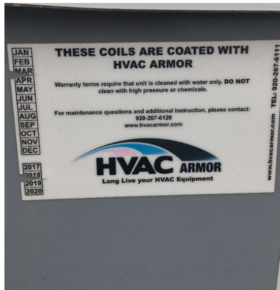
Figure 11: HVAC Armor tag on Roof Top Unit at City Hall
