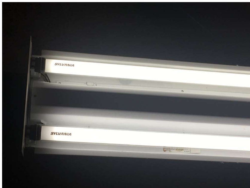
Figure 21: Additional image showing missing plastic cover
