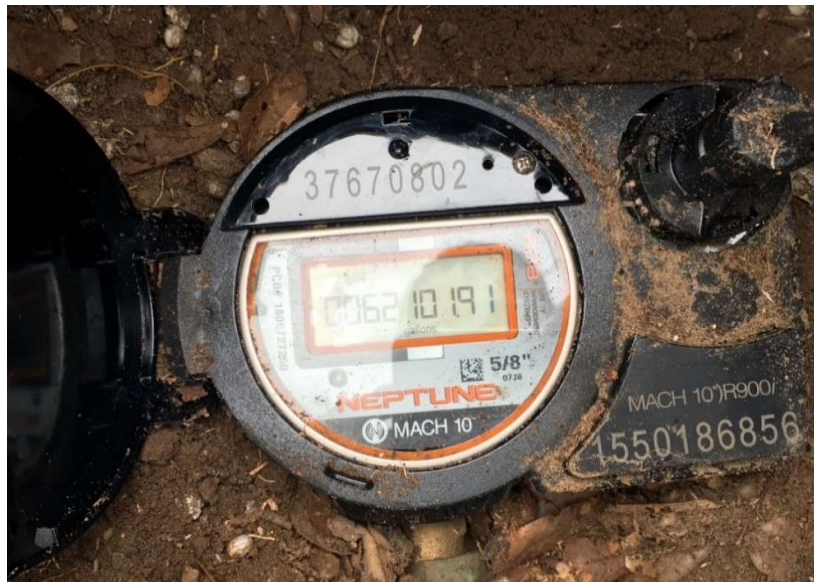
Figure 3: Typical 5/8" Neptune Mach 10 Water Meter in Service
