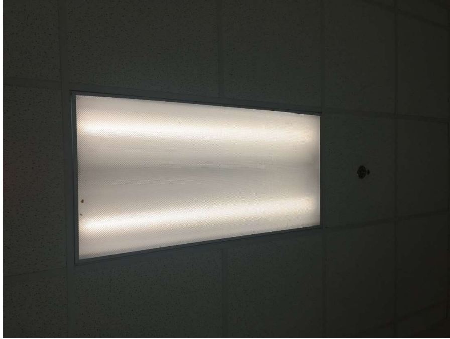
Figure 23: 2 x4 LED fixture at City Hall
