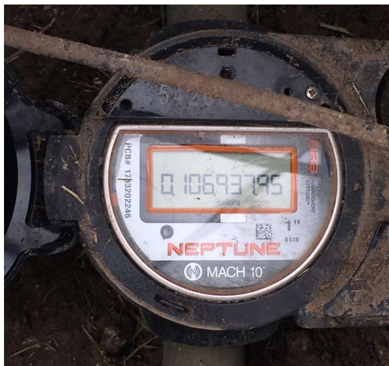
Figure 4: Typical 1" Neptune Mach 10 Water Meter in Service
