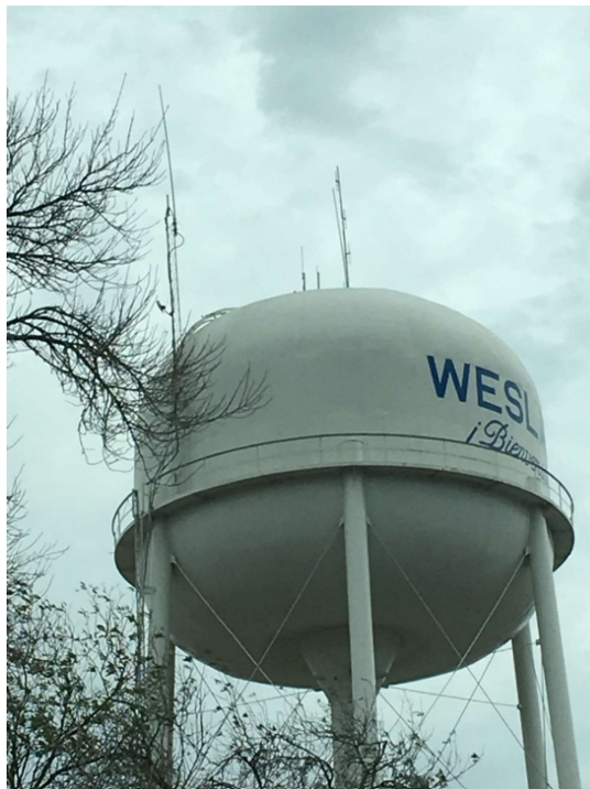
Figure 7: AMI Collector atop Water Tower
