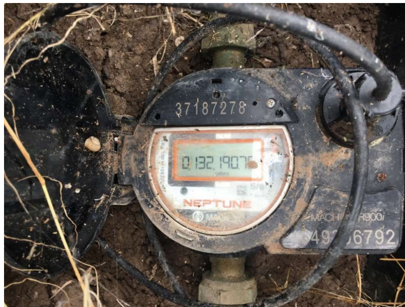
Figure 6: Typical 5/8" Neptune Mach 10 Water Meter in Service
