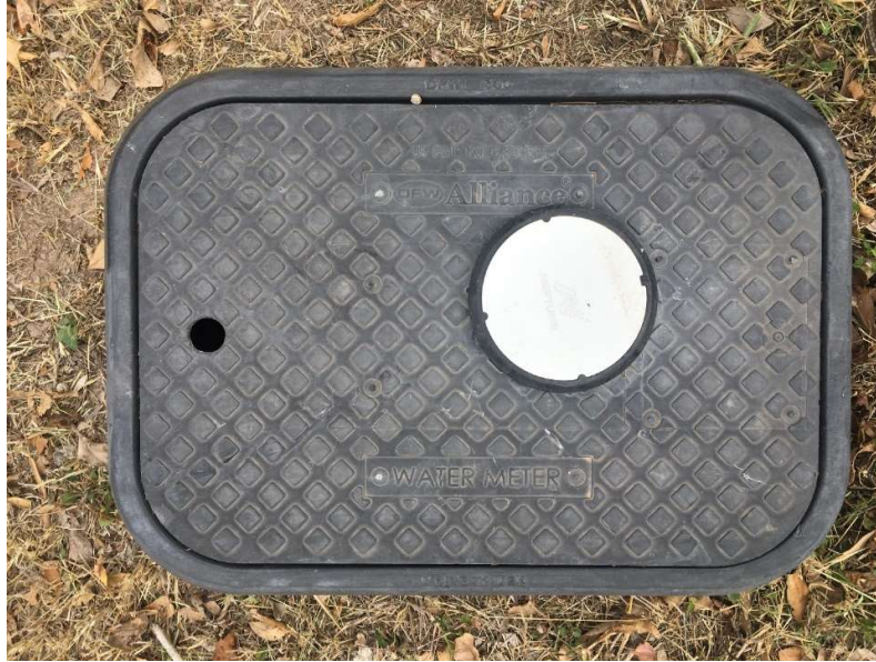
Figure 5: Typical Water Meter Lid & AMI Antenna in Service
