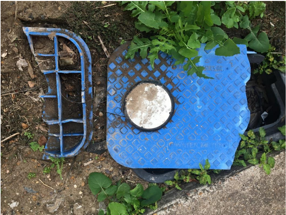
Figure 14: Broken Meter Lid
