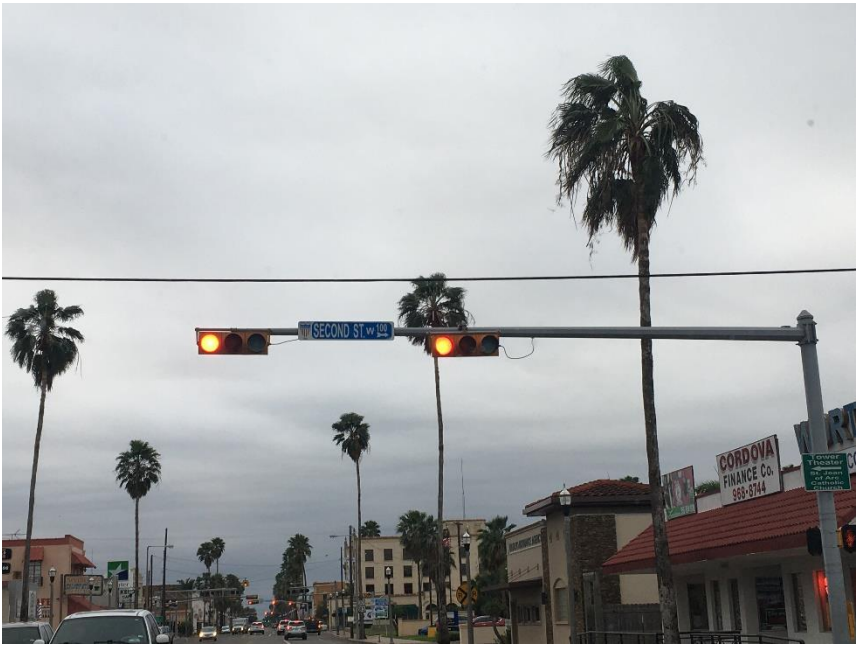
Figure 40: LED Traffic Signal
