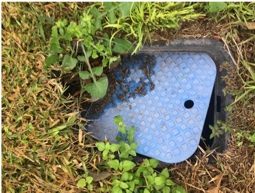
Figure 6: Meter Lid inspected was dislodge upon arrive, antenna was not flush with ground (Corrected after inspection)
