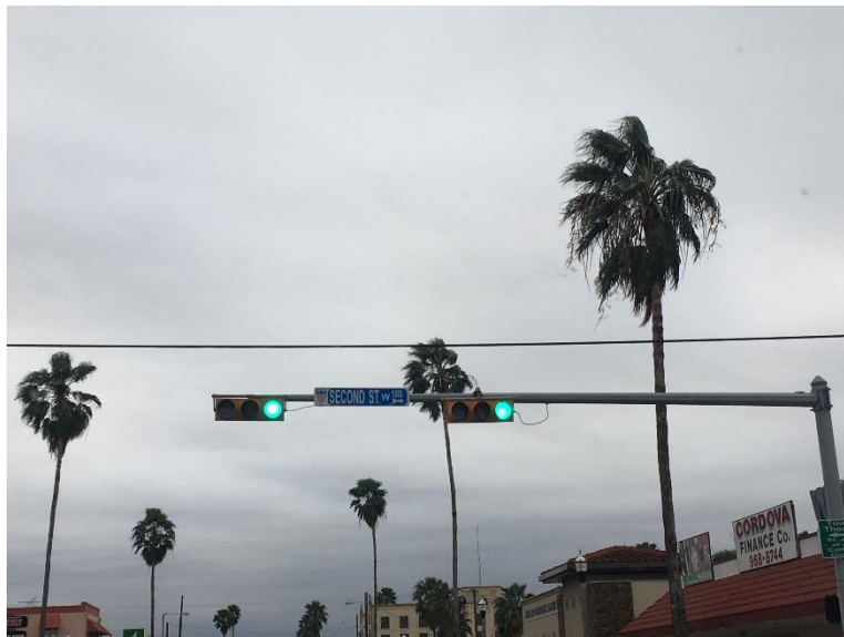
Figure 39: LED Traffic Signal
