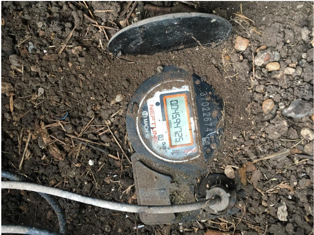
Figure 12: Typical 5/8" Neptune Mach 10 (Meter was covered by dirt)
