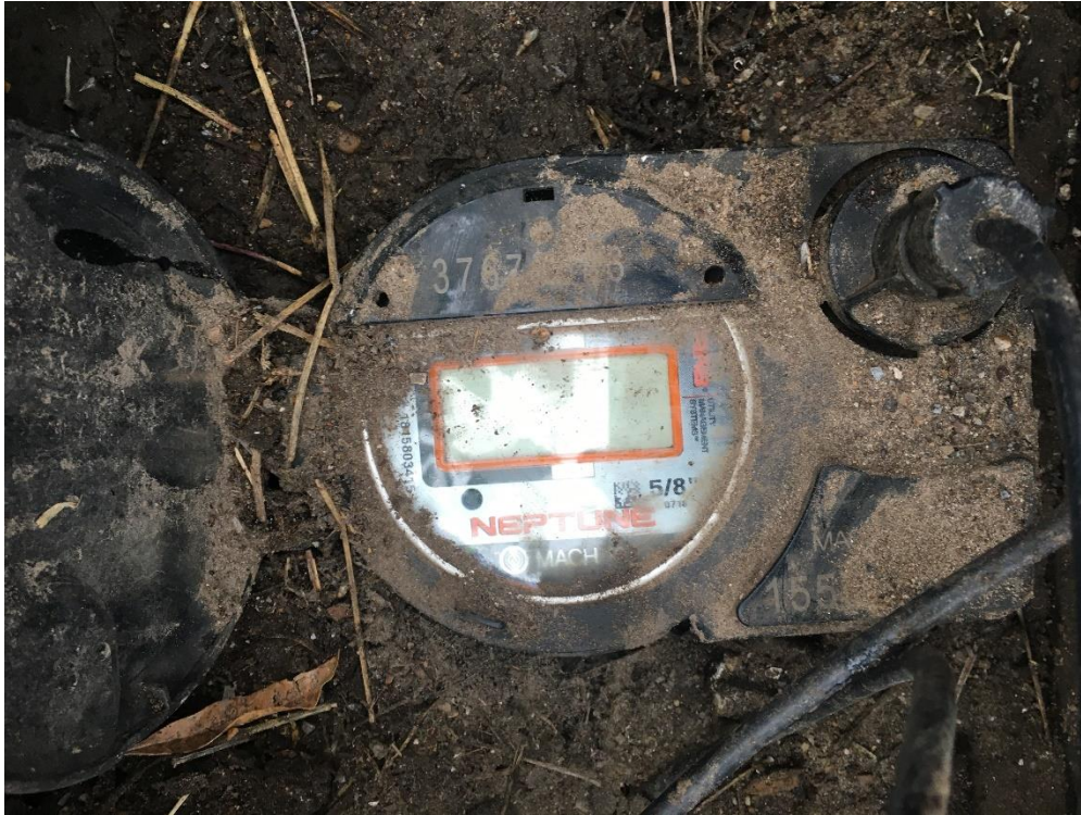
Figure 5: Typical 5/8" Neptune Mach 10 meter (Meter was covered by dirt)
