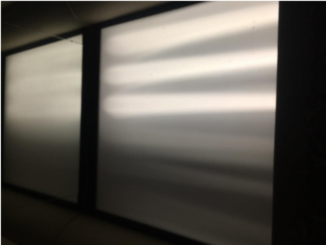
Figure 35: Additional image burned out LED lamps
