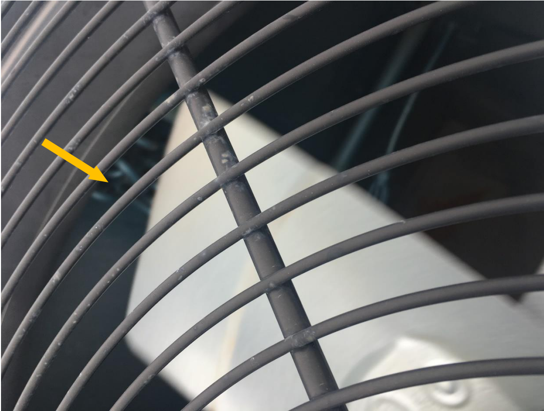
Figure 17: Roof Top Unit Coils sprayed with HVAC Armor
