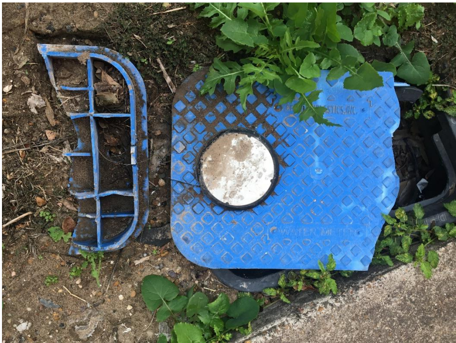
Figure 14: Broken Meter Lid
