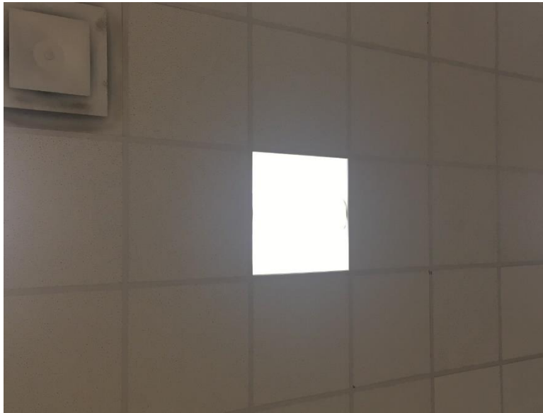
Figure 28: 2x2 LED Light Fixture at Public Library
