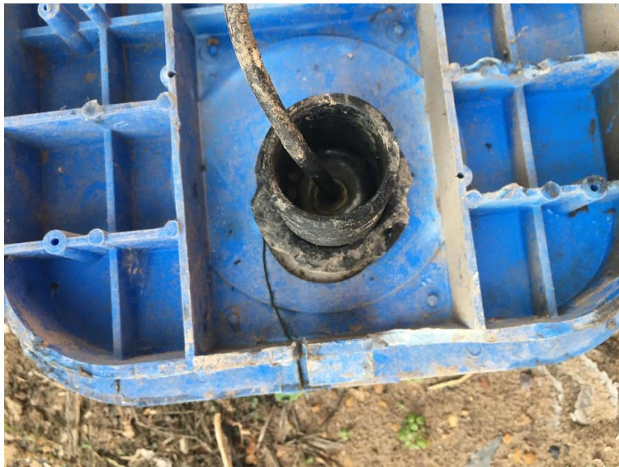
Figure 4: Inspected Meter Lid (lid was damaged around the antenna bracket)
