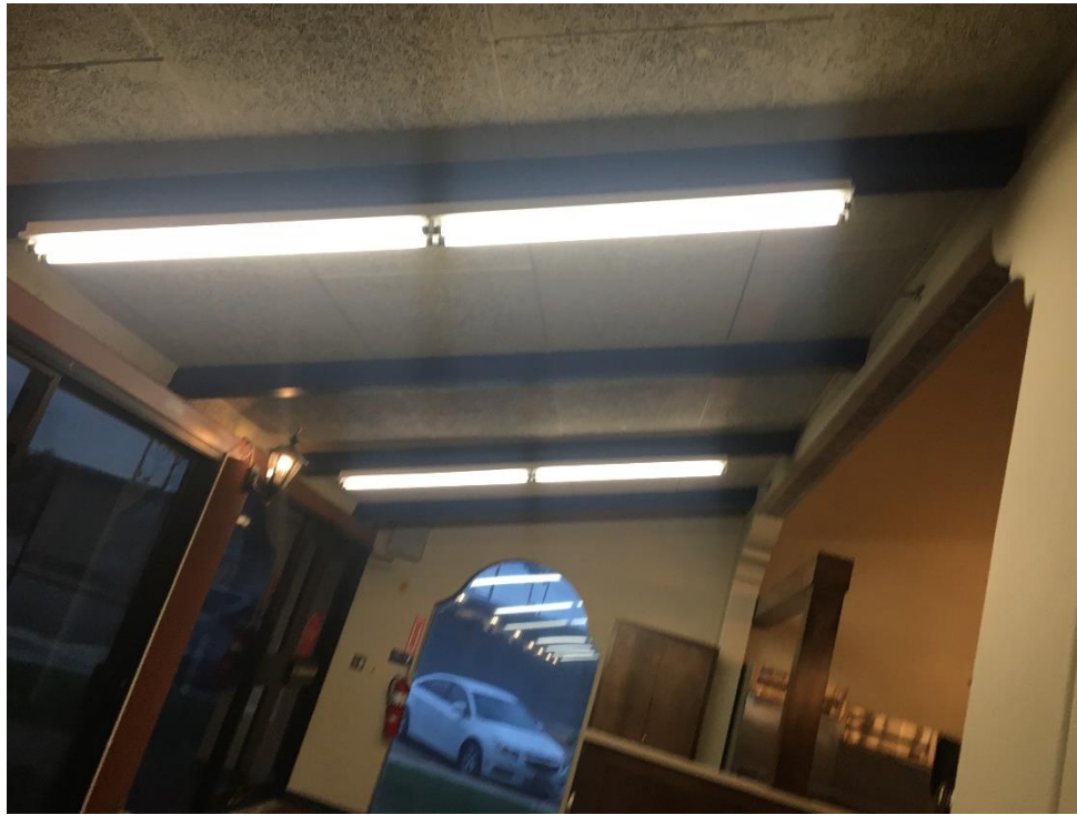
Figure 38: Public Library LED fixtures with Plastic Protective Sleeves
