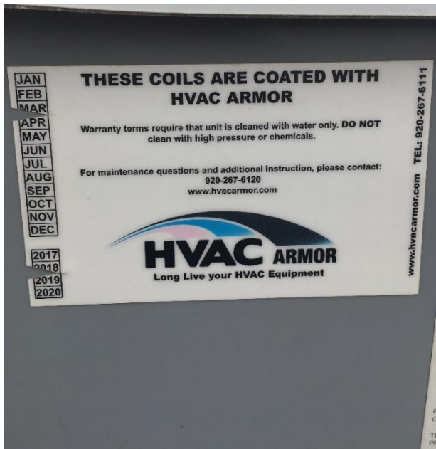
Figure 19: HVAC Armor tag on Roof Top Unit at City Hall
