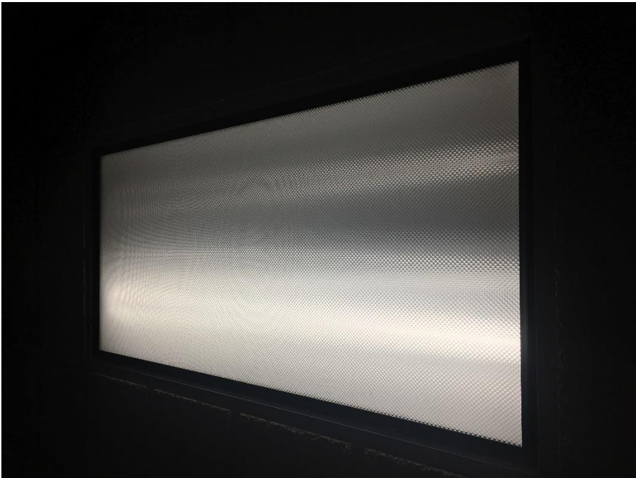
Figure 34: Public Library LED Fixtures with burned out lamps (Elevator Area)
