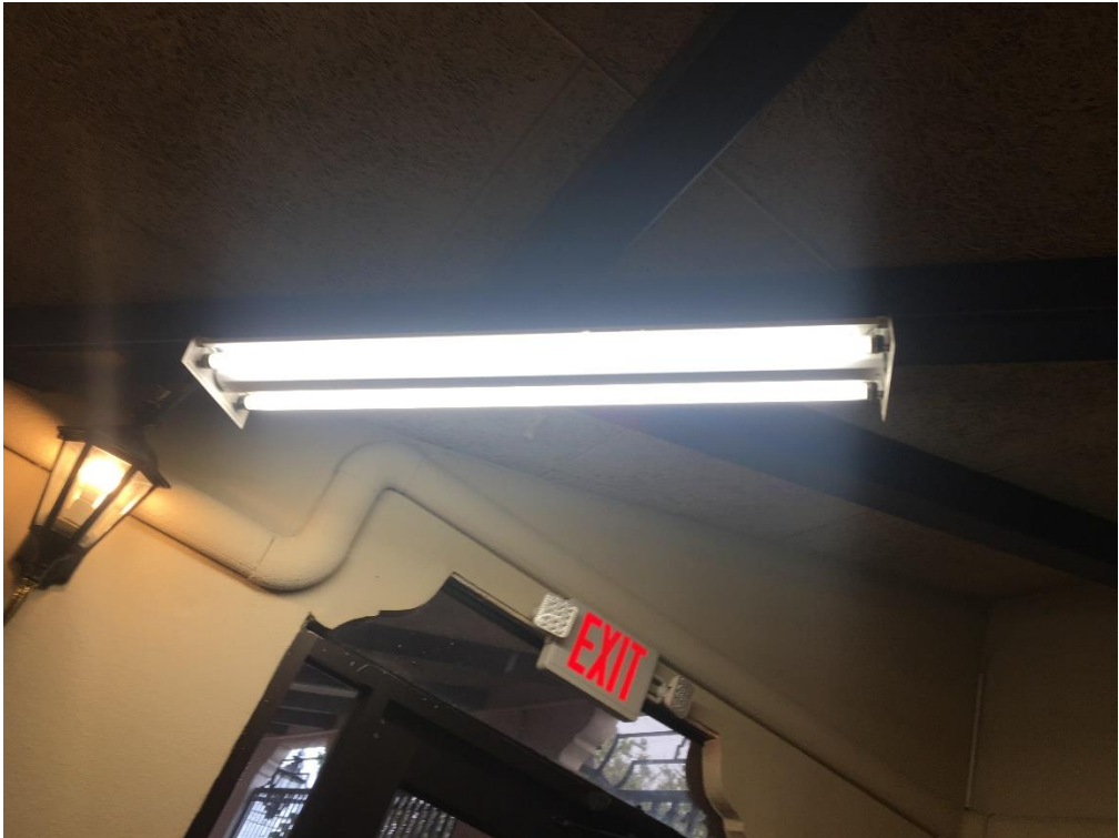
Figure 33: 2x4 LED Light Fixture at Public Library with Plastic Protective Sleeve
