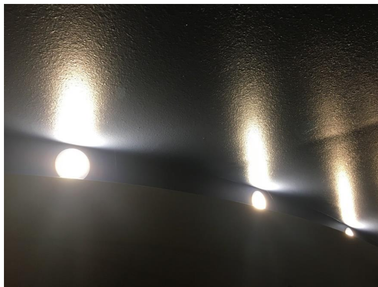
Figure 29: Accent LED Lighting at Public Library
