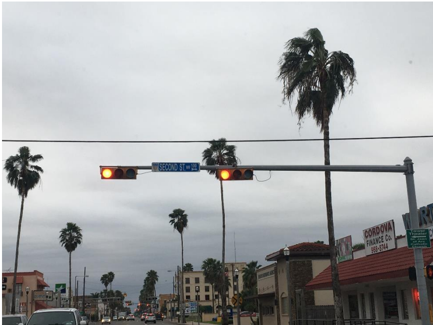
Figure 40: LED Traffic Signal
