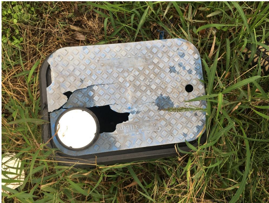
Figure 11: Damaged Meter Lid (possibly impact around meter antenna)
