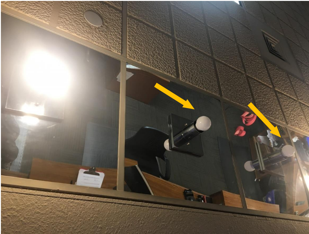
Figure 36: Image from Year 1 shows in-operable Screw-in LED lamp
