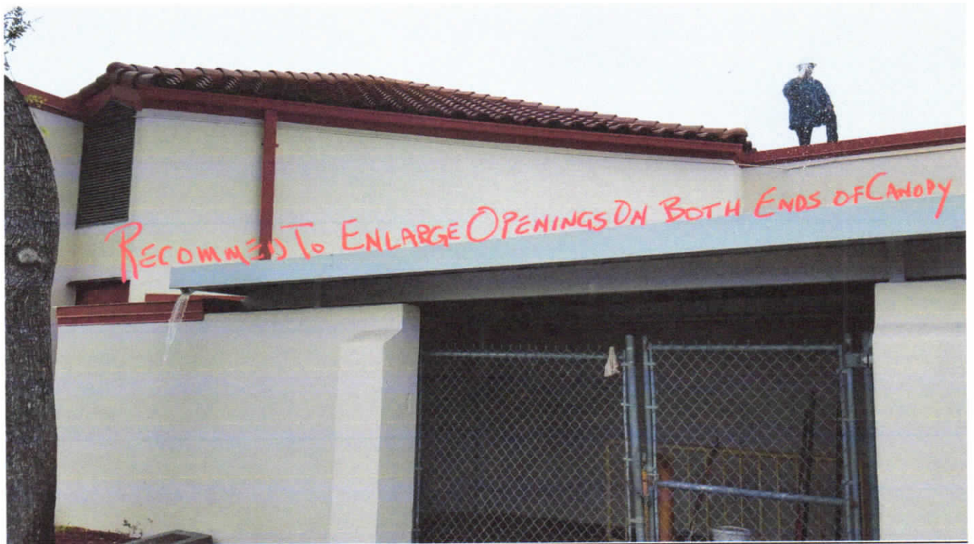
PHOTOGRAPH 3: Small openings in the canopy gutter are susceptible to becoming obstructed with debris.
