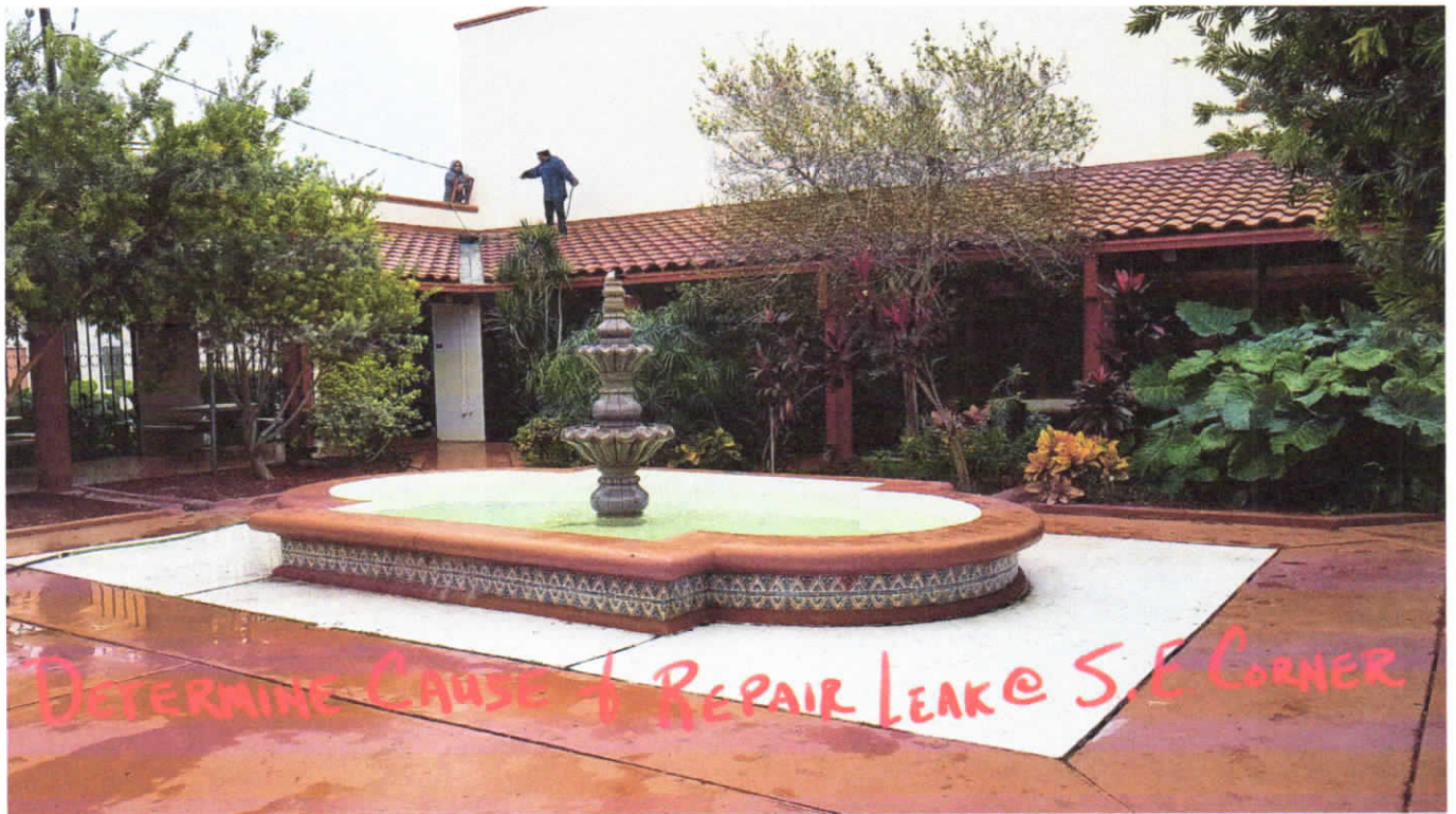
PHOTOGRAPH 1: Water test produced a leak in the Library that would be near the S.E. corner of the Courtyard.
