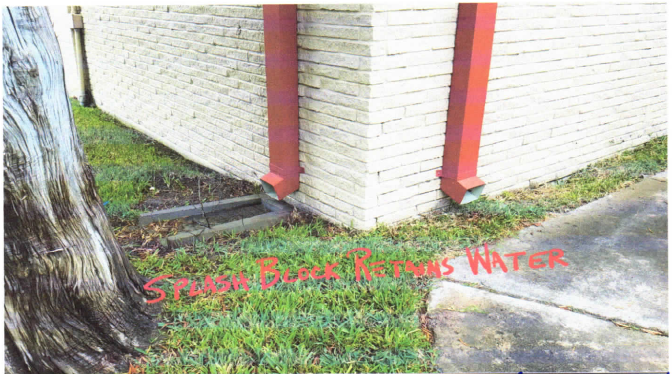
PHOTOGRAPH 4: Some of the splash blocks appear to retain water but, should drain to the outside.
