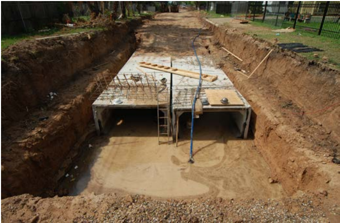
Image 2.2 | Stormwater infrastructure | CURPR
