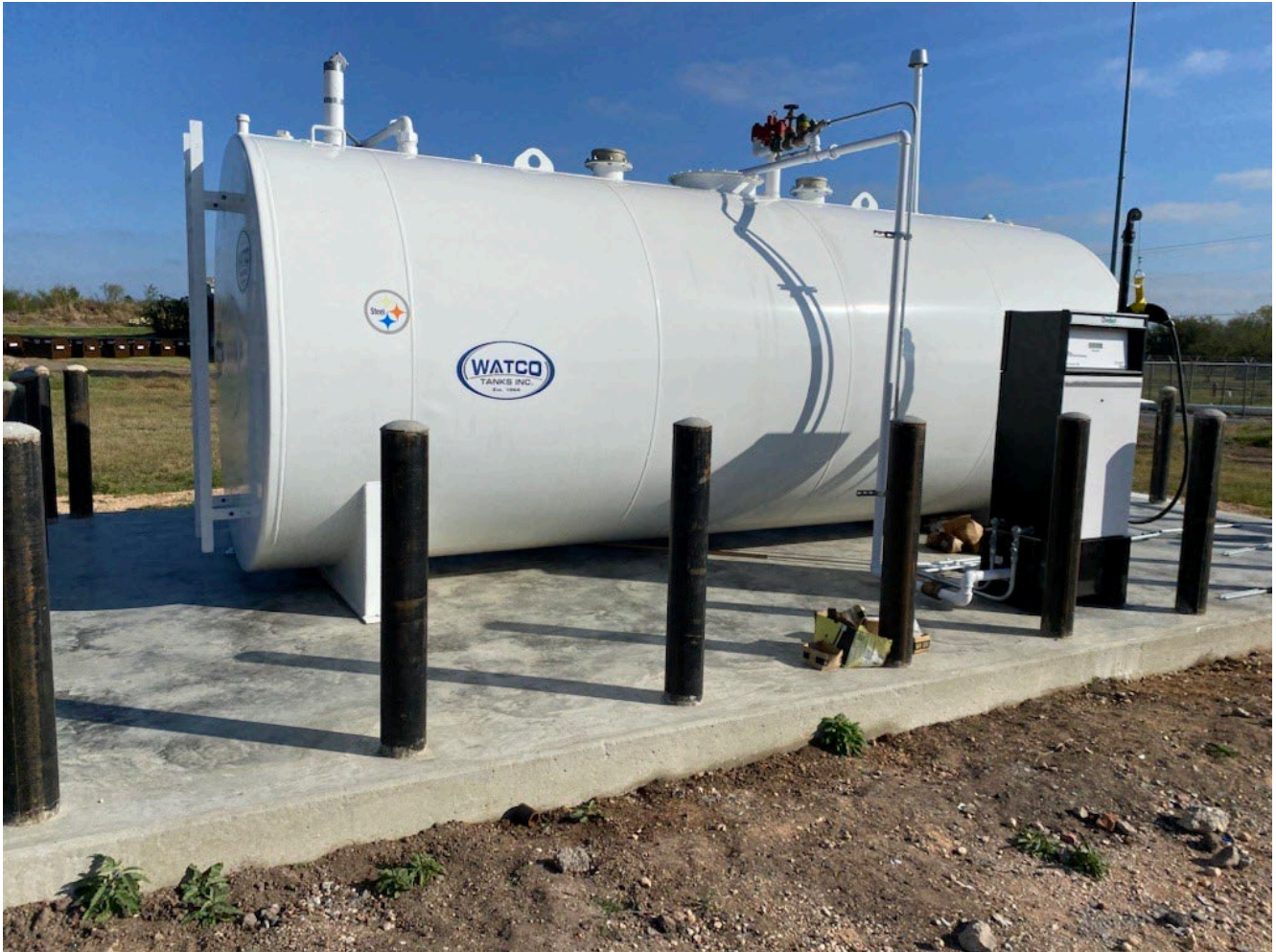
This is a Diesel only tank 8,000 gallon capacity located at 3000 S. Border Ave. Weslaco, Texas
