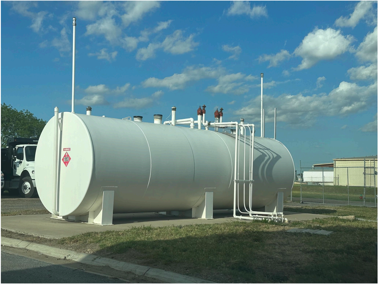
This is the Unleaded and Diesel split tank located at Public Works Warehouse 1912 Joe Stephens Ave. Weslaco, Texas 6,000 gallon Unleaded 4,000 gallon Diesel
