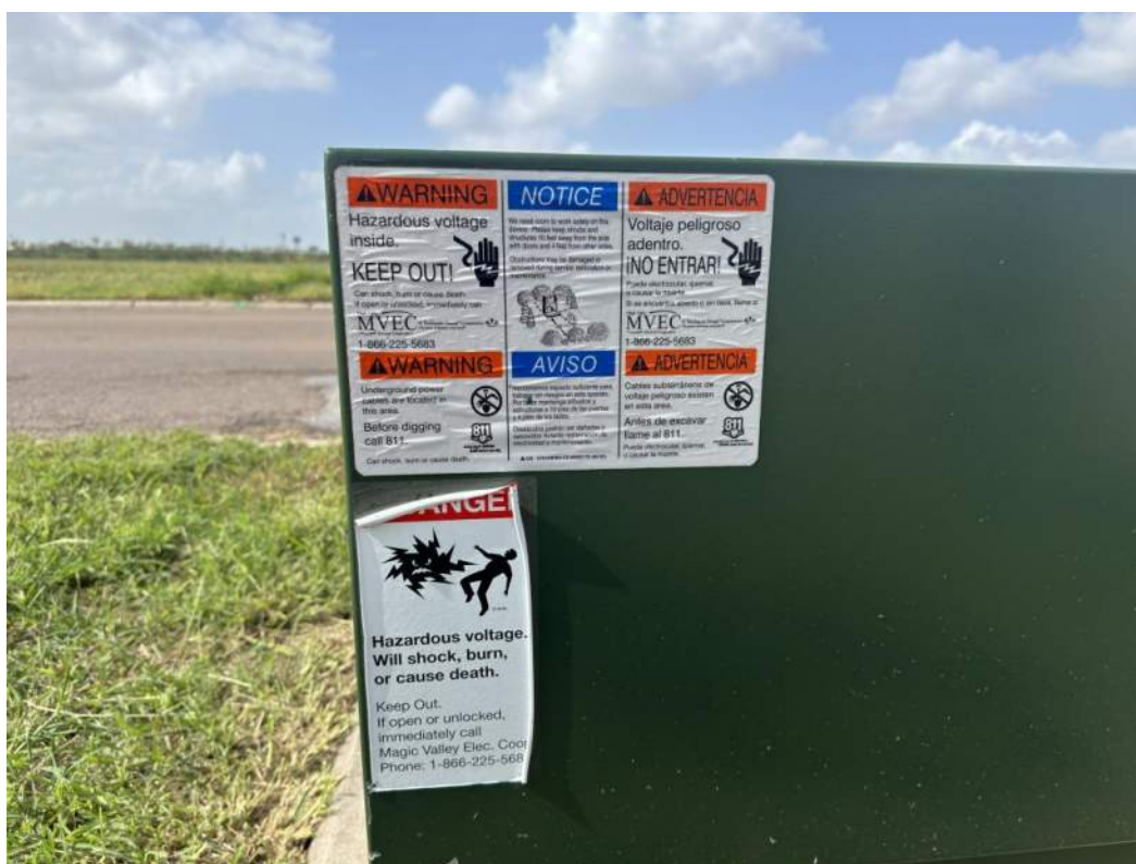
Photo 6: Northeast corner of Vo Tech Dr. and E. Pike Blvd facing South (Close up of warning labels on presumed transformer)
