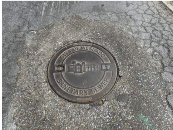
Photo 7: Vo Tech Dr. and E. Pike Blvd facing North (Sanitary manhole cover)
